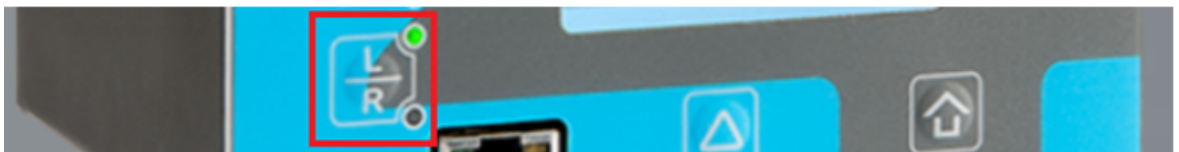
The Local/Remote switch at Local mode
